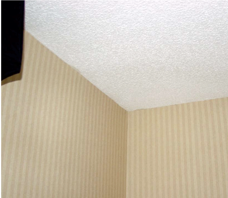
Figure 2a) Visual image with no visible signs of mold.
